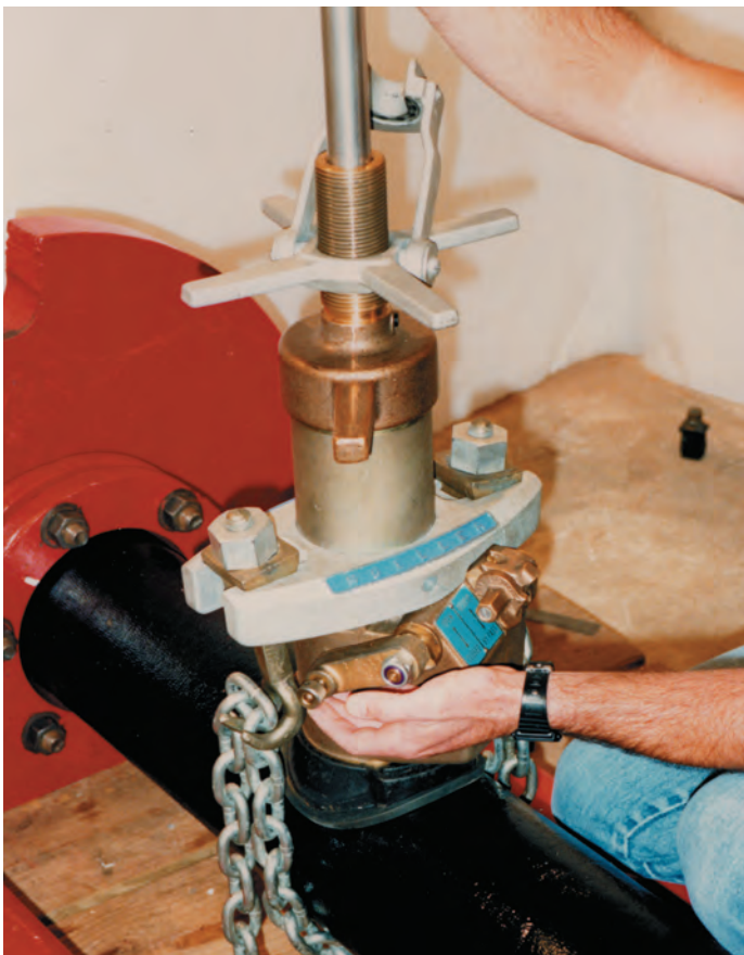
Each material was tapped according to recommendations. The average time to tap Ductile Iron (above) was 16 minutes.
