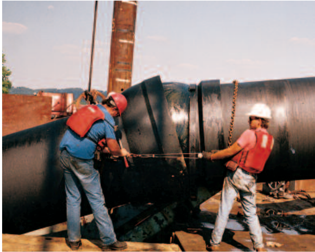
Above: Workers use come-alongs while installing Ductile Iron pipe with boltless ball and socket joints. These joints consist of a precision-machined ball that fits into a precision-machined socket, a rubber gasket that provides a pressure-tight seal, and a retainer ring that provides longitudinal restraint. The joint is leak-free throughout the full range of deflection.
