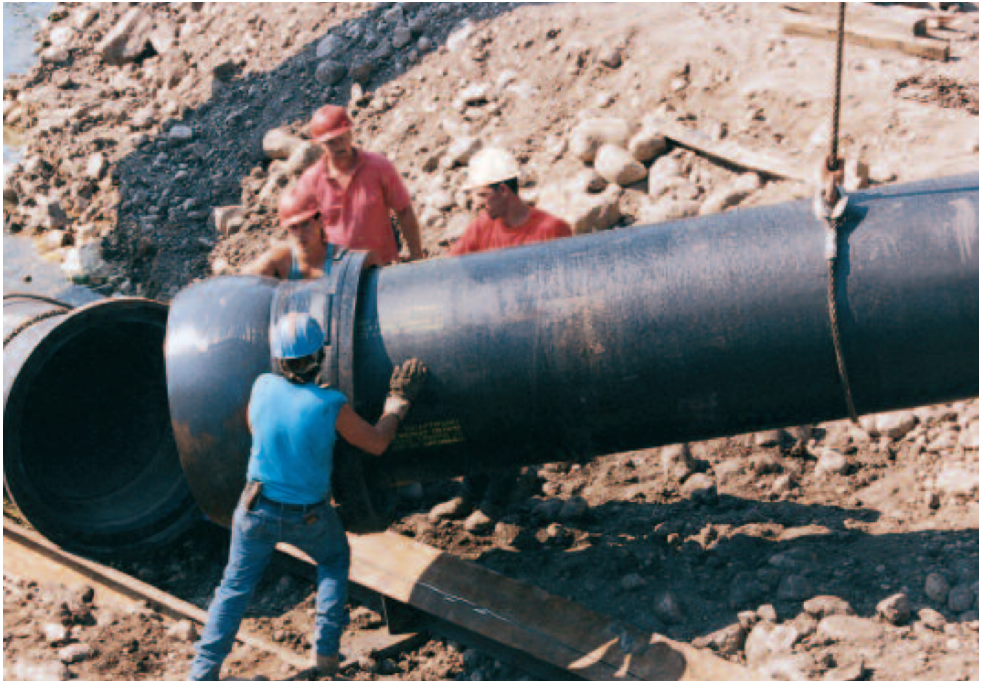
Below: In many subaqueous installations, the majority of the assembly can be done on dry land. Here, a crew lowers a piece of Ductile Iron pipe into place on top of a launching ramp from which cables will pull it across the water.
