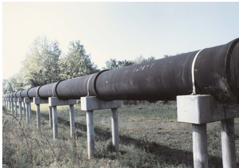
Ductile Iron is well-suited for use in pipe-on-supports applications due to its tremendous beam strength.
